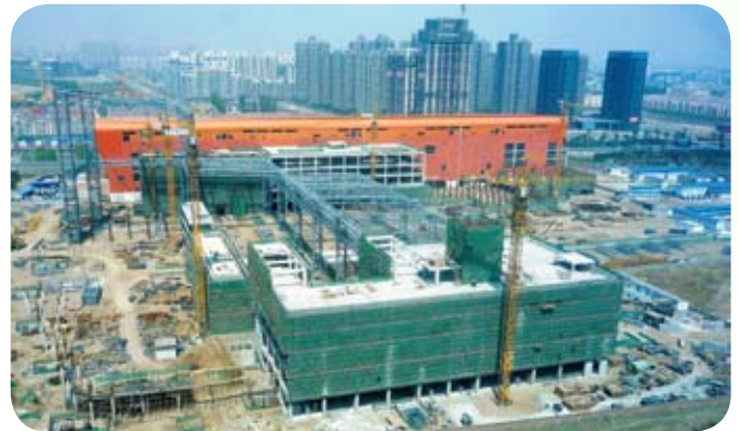
Aerial view of Phase 1 of Great Mall of China - Construction in progress.
