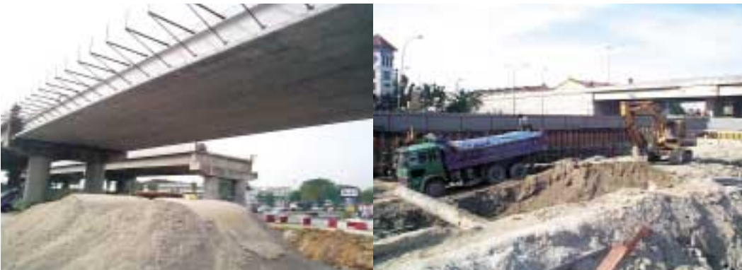
Excavation works for the 2nd phase of the PJS 8 underpass at Bandar Sunway.
